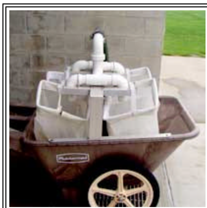
These filters capture grass clippings, dirt, fertilizer and other contaminants from the reclaimed water before it is recycled.
