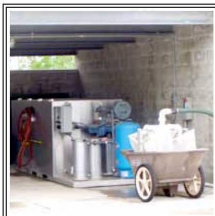
The Detroit Lions' Practice Facility was designed to be environmentally responsible. This water recycling station cleans and filters the water used to clean mowers and vehicles.
